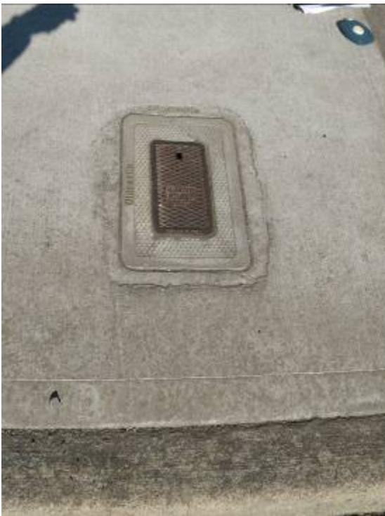
Water meter will remain.
